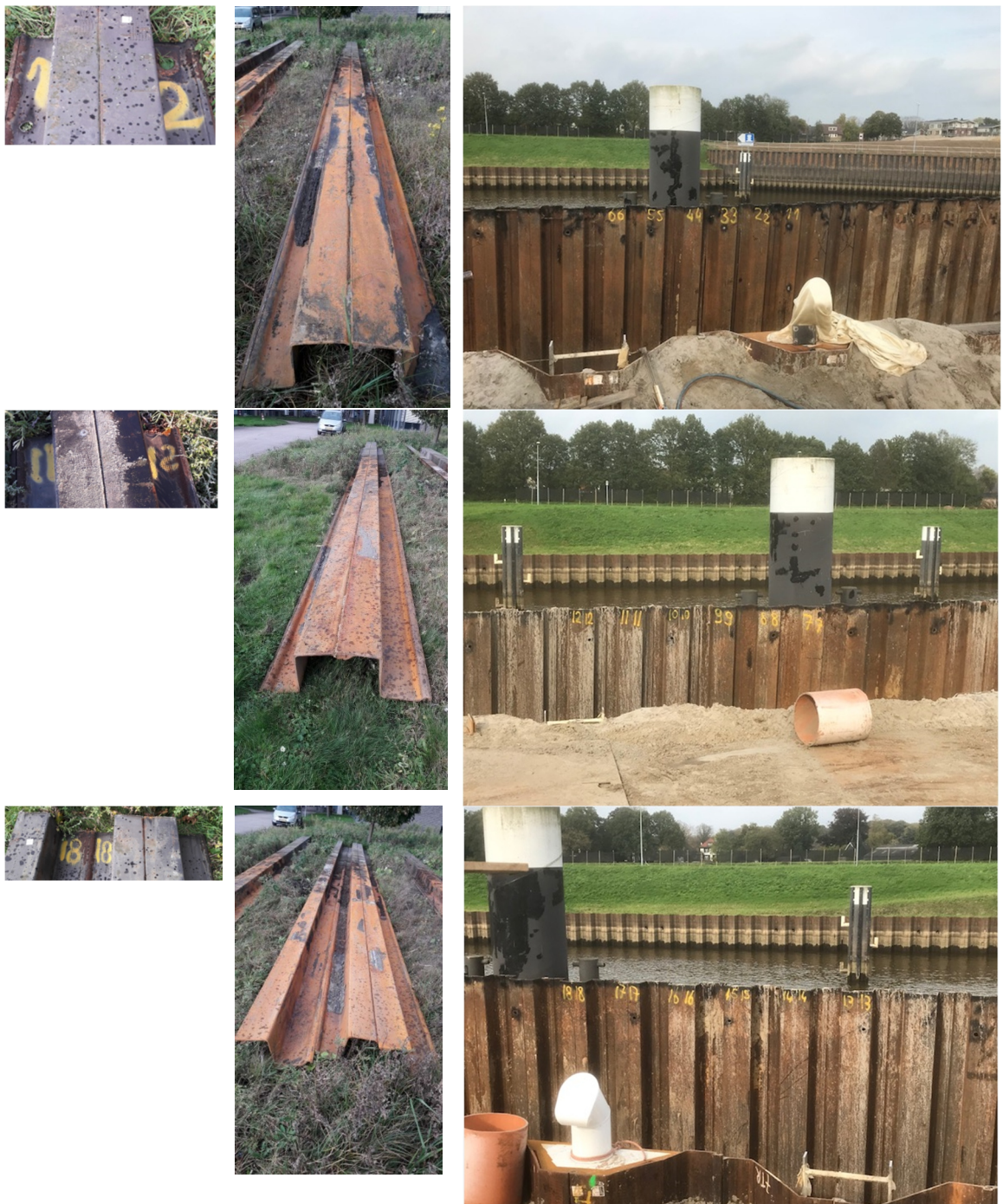
Figure 1.2 Eefde sheet piles Right: The 37 sheet piles sections just before extraction in October 2017 the photos are taken from landside (standing on top of the new sheet pile wall, the soil between old and new sheet pile wall is already excavated). Middle: the waterside of the 3 sets of sheet piles (in total 7 sheet pile sections) (before cleaning) transported to Deltares Left: top of the 3 sets of sheet piles at the Deltares, the photos are made of the waterside
