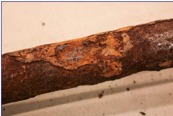
Figuur 76 Corrosie product detail anker Loofr-2.
