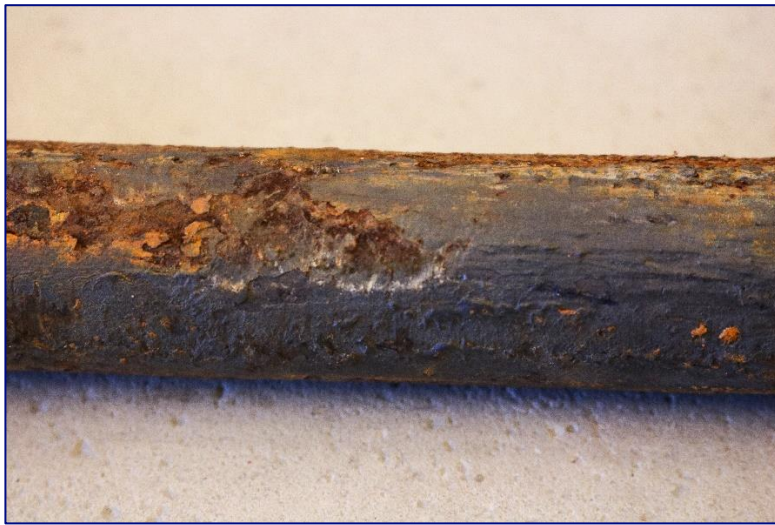
Figuur 69 Corrosie product detail anker locatie II.
